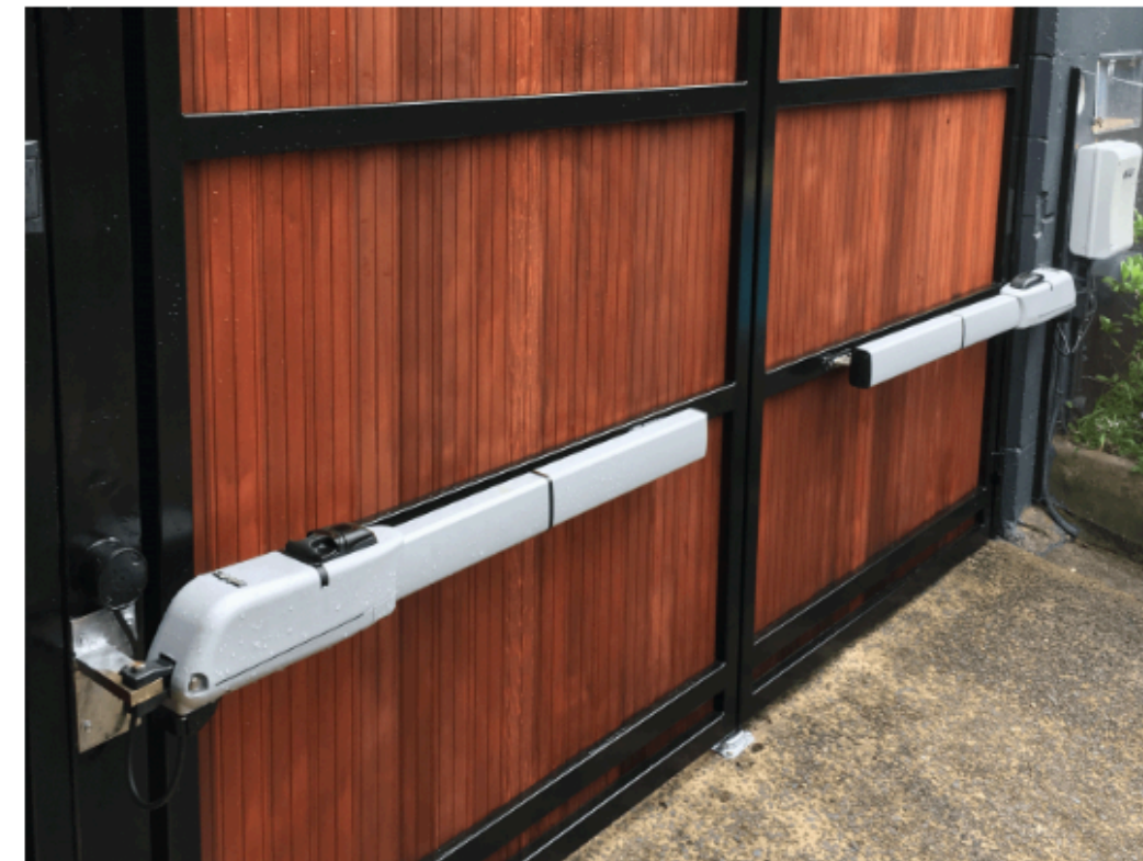
Swing Gate Automation
